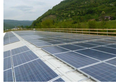
Location: Cuneo, Italy Project Type: Roof Top Project Scale: 1.8 MWp
