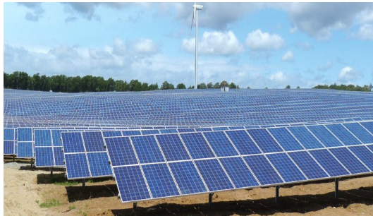
Location: San Floro, Calabria, Italy Project Type: Ground Mounted Project Scale : 24 MWp
