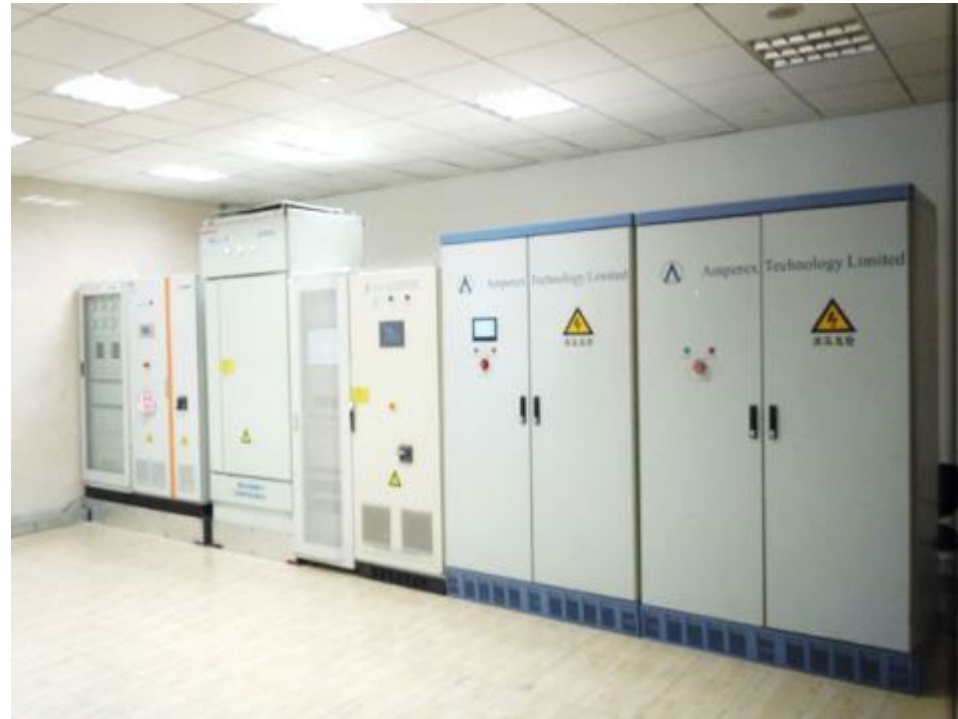
Capacity : 100 kW / 200 kWh Type: PV + Storage + Diesel
