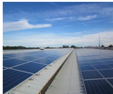
Location: Campania, Italy Project Type: Roof Top Project Scale: 1,8 MWp
