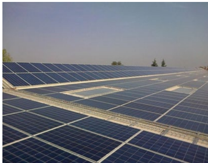
Six Energy Location: Emilia Romagna, Italy Location Type: Roof Top Project Scale: 2,3 MWp
